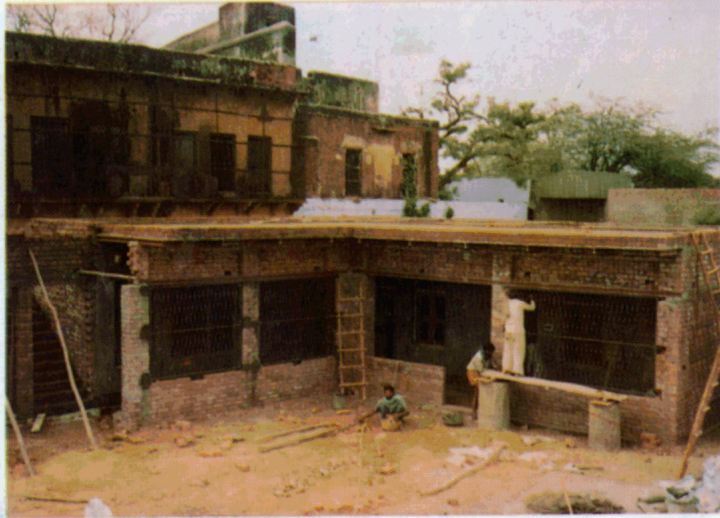
left: At Śrī Vṛndāvan, Śrī-Rūpa-Sarasvatī-Śrīdhara Sevākuñj under construction, 22nd January, 1996. [see front page 'Āchāryadev's Triumphant Entrance to Holy Vṛndāvan Land']
